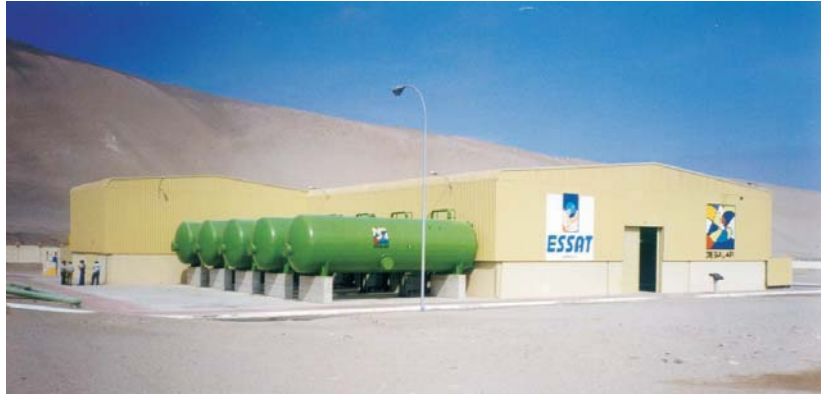
General view of the plant
